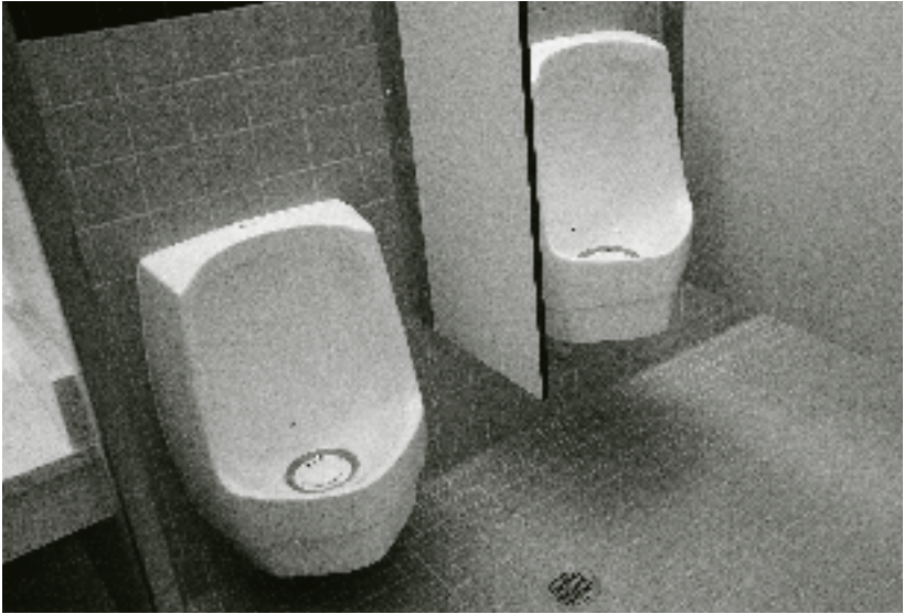
Water consumption in the bathrooms is reduced with the use of waterless urinals, 1.6-gallon flush toilets and low-flow bathroom faucets that shut off automatically. PHOTO: TIM DAVIS
