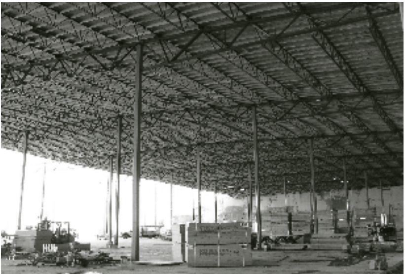
Interior columns and roof structure contain recycled steel, and almost all of the wood products used in construction are certified by the Forest Stewardship Council. PHOTO: JANE DAY
