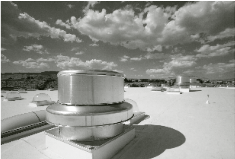
A night-flush exhaust system on the roof replaces the hot air of day with cool nighttime air, thereby eliminating the need for air conditioning. PHOTO: TIM DAVIS
