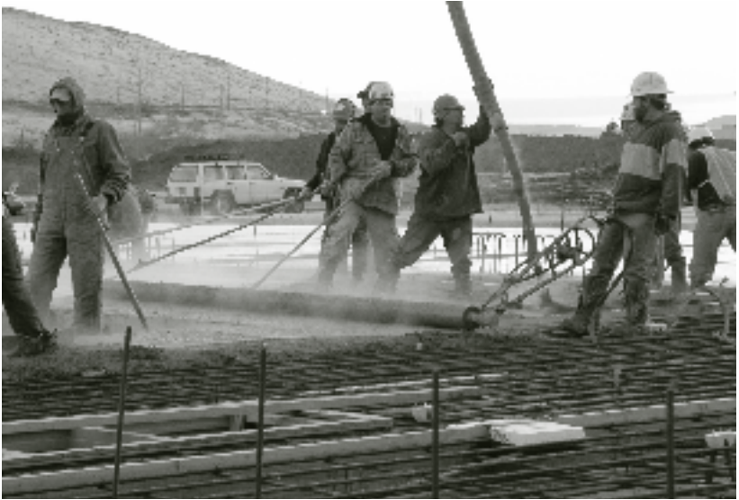
Concrete walls and floors contain recycled content, including steel rebar and flyash. PHOTO: JANE DAY
